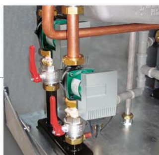
Pumps and gate valves
